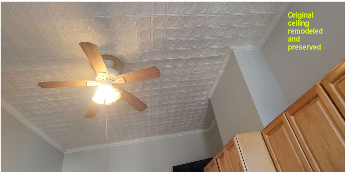
1st floor front. Used as a Day Care center. Note the 12 ft ceiling
